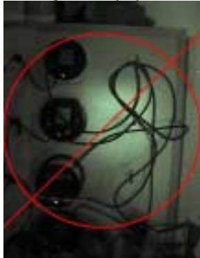
Fig. 4.4. Tangled cox box cables
